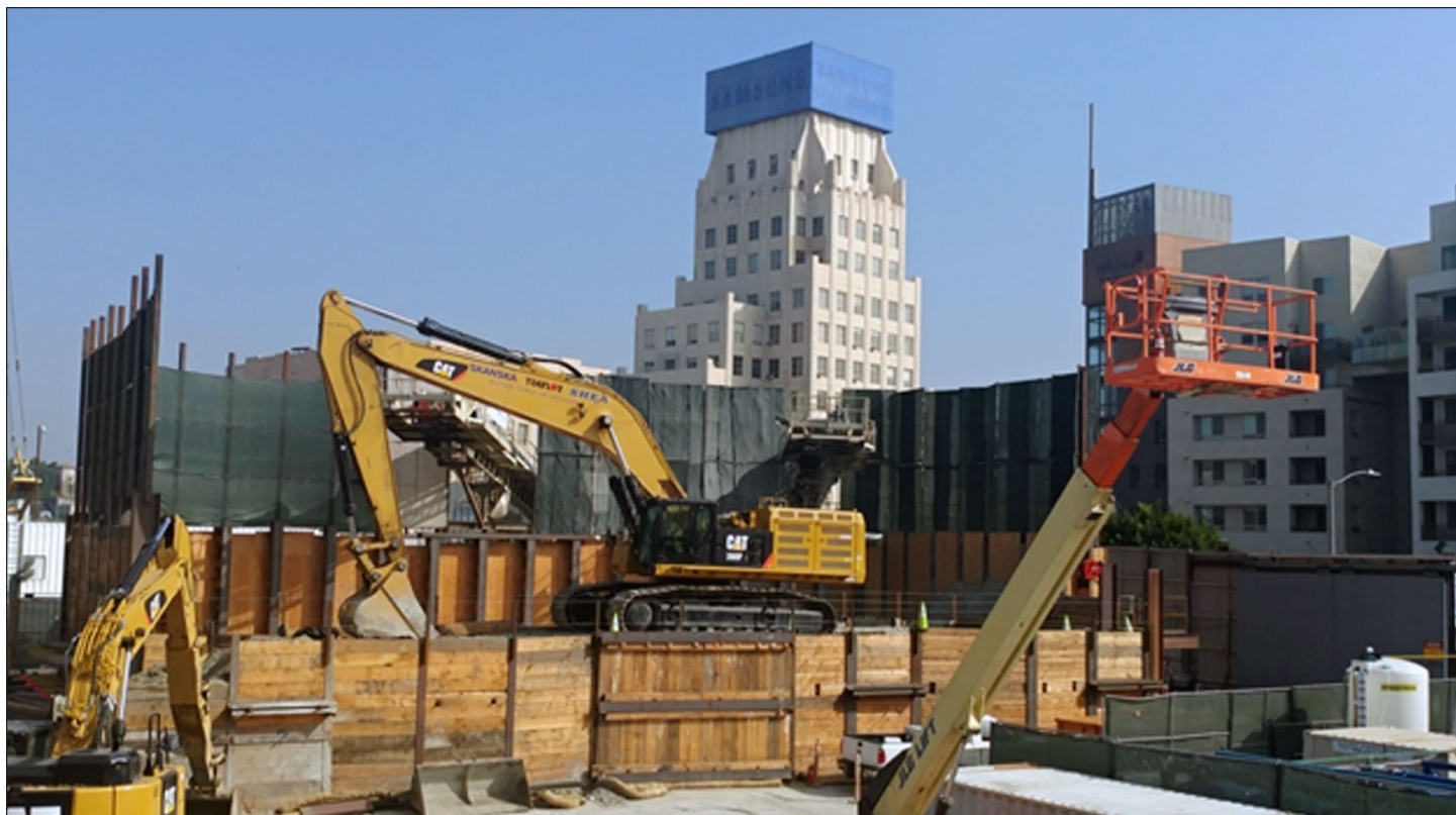
Figure 4: Staging and Construction Site for the Purple Line Extension in Los Angeles, California
